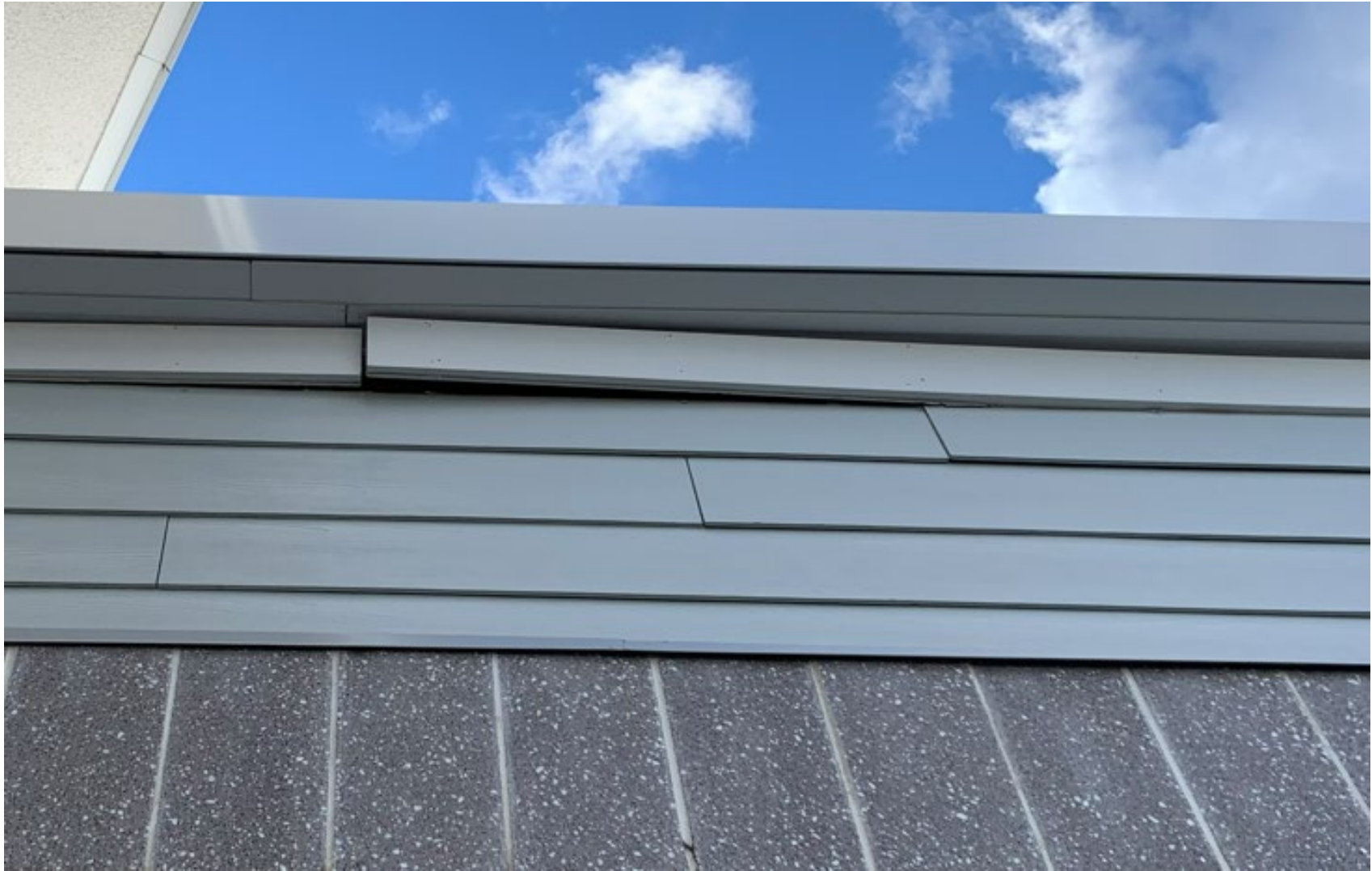
Example of trim board not secure do no blocking or stud , remove trim board ,install blocking , reinstall
